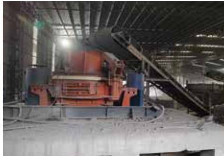
Hunan Limestone Project, Capacity: 500 tons per hour
