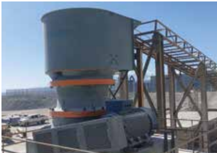
Gansu Limestone Project, Capacity: 800 tons per hour
